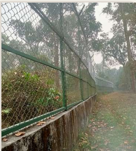
Vertical extension for existing herbivore fencing for conversion to carnivore boundary fencing (L-1300.00 m at NBWAP)
